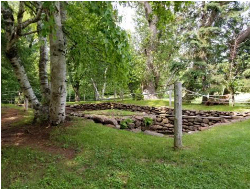
The cellar and foundation of L.M. Montgomery's childhood home in Cavendish, Prince Edward Island. The original kitchen, which had been elsewhere, was returned to the site in late 2018. Photo by Caroline Jones, 2018.
